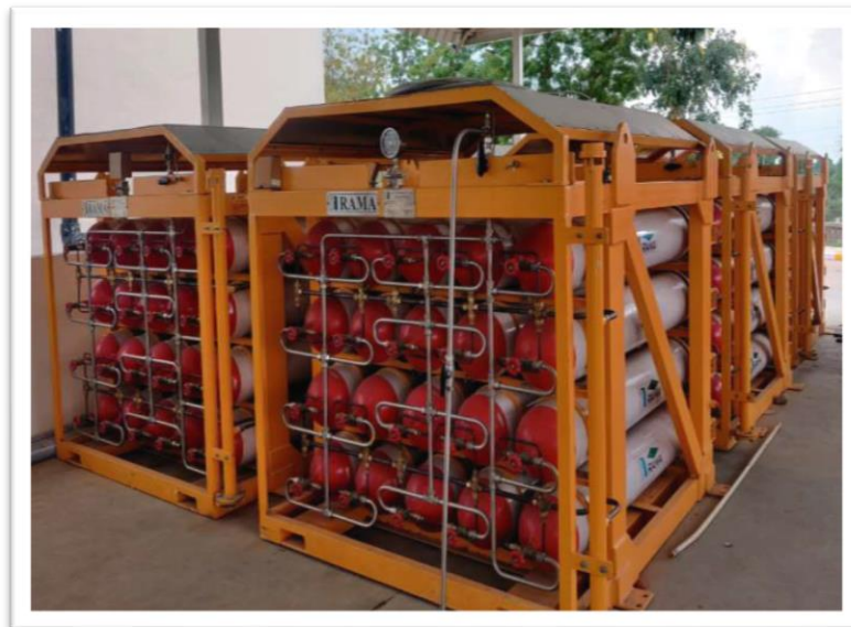
Compressed purified gas is store in the Cylinder Cascade system Storage Pressure: 250 Bar
